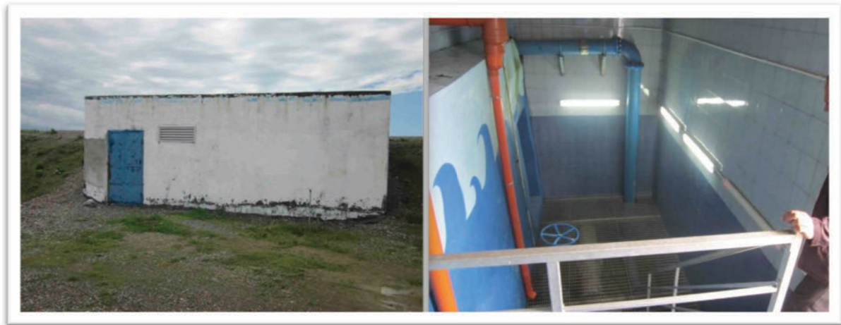
Picture 4: Outside and Inside of one of the four control rooms (outlet chamber) (Photo: C. Stubenberg)
