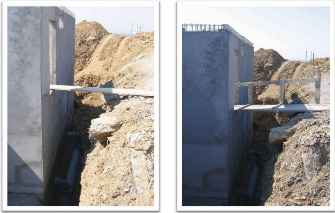
Picture 24: Wooden Bridge with and without safety measure. (Photo: ADA Project Archive)
