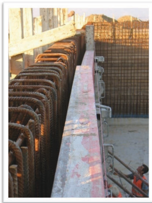
Picture 23: The Reinforcing steel-bars installed in the formworks. (Photo: ADA Project Archive)
