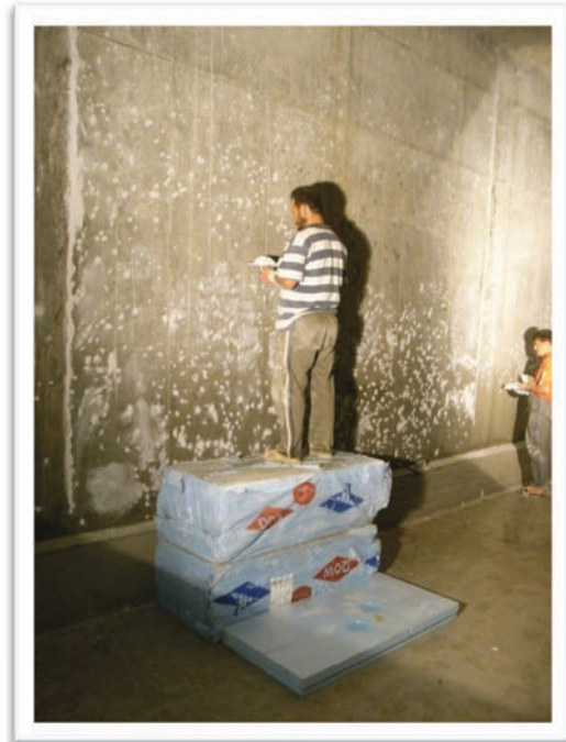
Picture 27: Workers closing pores with special cement inside the reservoir (Photo: ADA Project Archive)
