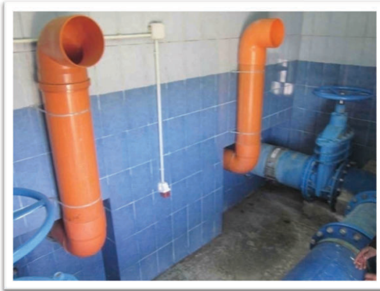
Picture 13: Orange aeration pipes and gate valves inside an inlet chamber.
