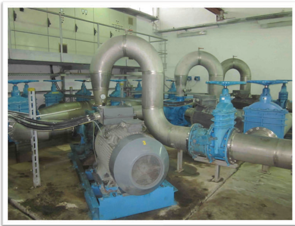
Picture 6: Pumping Station in the well-field, pushing water into the network and onto the Tepe hills.(Photo: C. Stubenberg)
